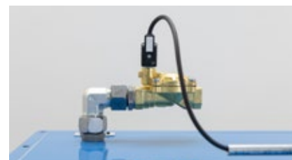
Inert gas connection
